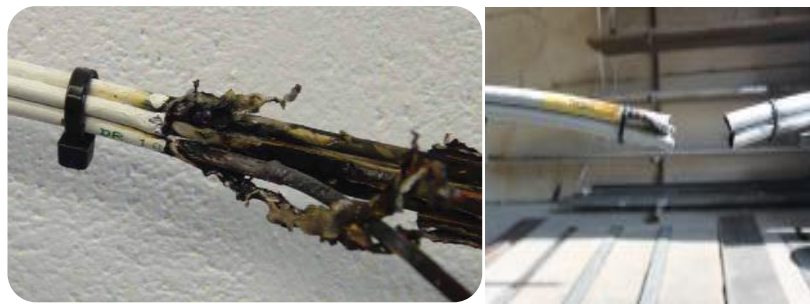
Figure 2.3-1 - Arc tracking and different power levels: 270 V (left) vs 3000 V (right)
